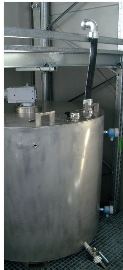
Resin tank and mixer
