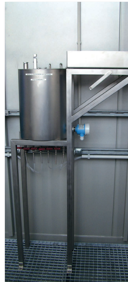
Peroxide tank with level control
